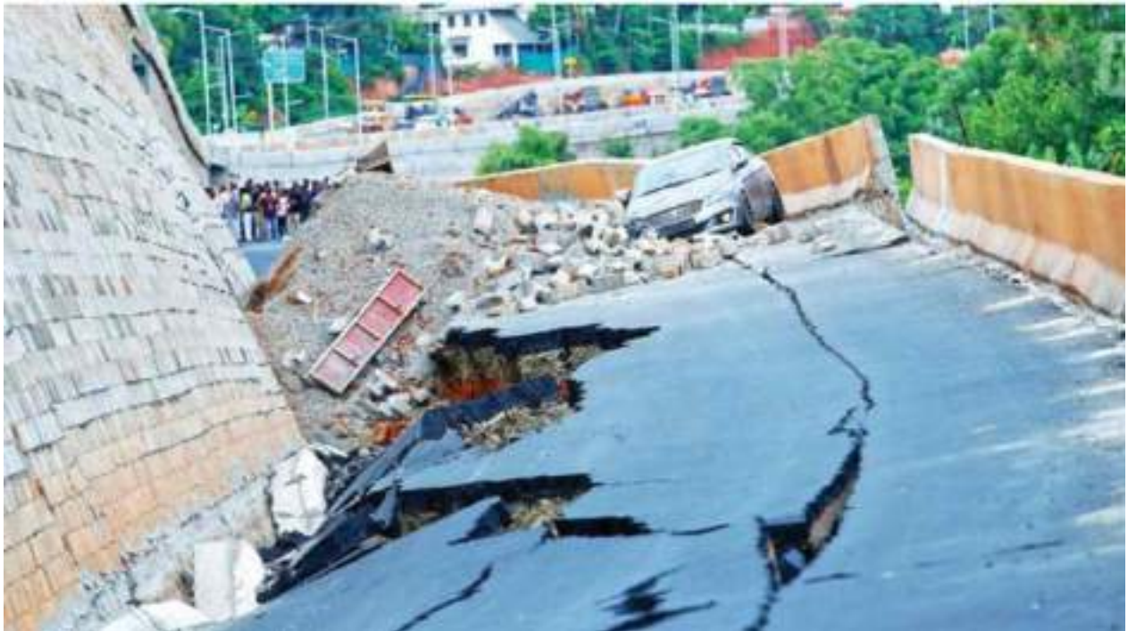
Fig. 1 NH-66 collapse in Malappuram
